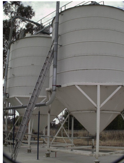
Typical bulk storage silos.
